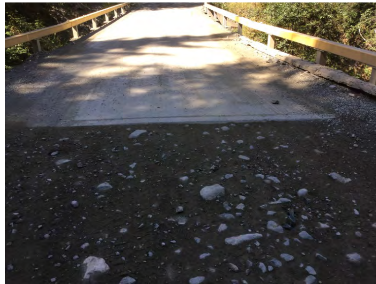
Potholes at approaches
