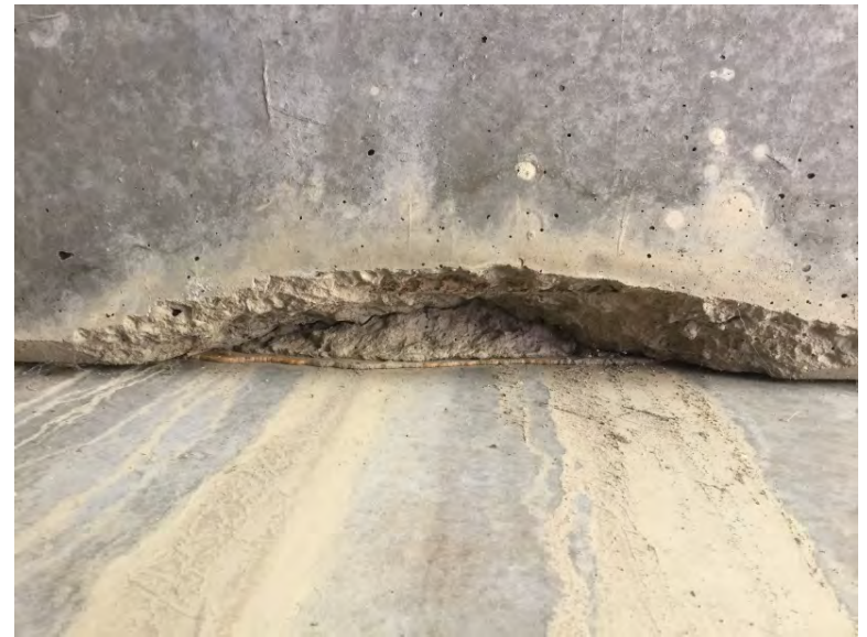
Left bank panel 1 damage
